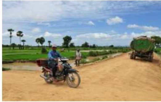
A villager rides his motorbike across a newly renovated road in Takeo province in southwestern Cambodia. The road was built under the Inter-Commune Cooperation scheme being piloted in 12 provinces in Cambodia.
